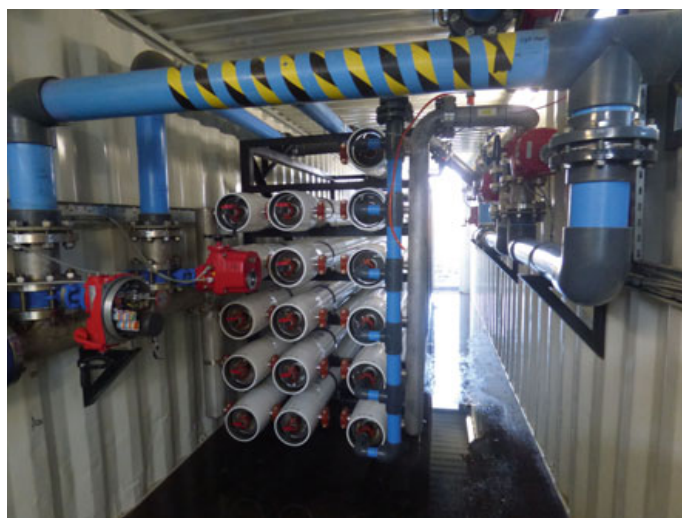
Fig. 5 Reverse osmosis plant
